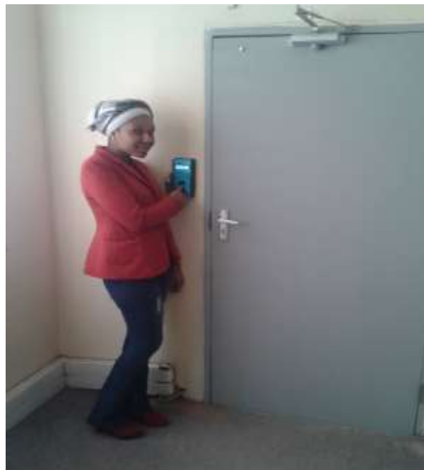
Fig 4 : Showing server room after installation of Suppression and Biometric System
